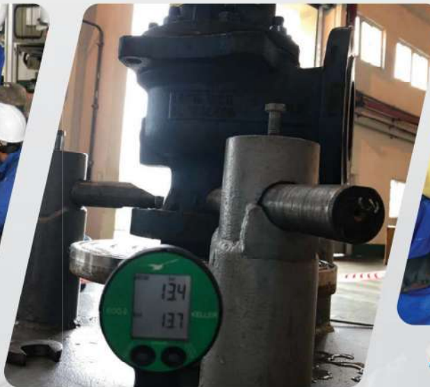
SAFETY VALVE OFFLINE TESTING
